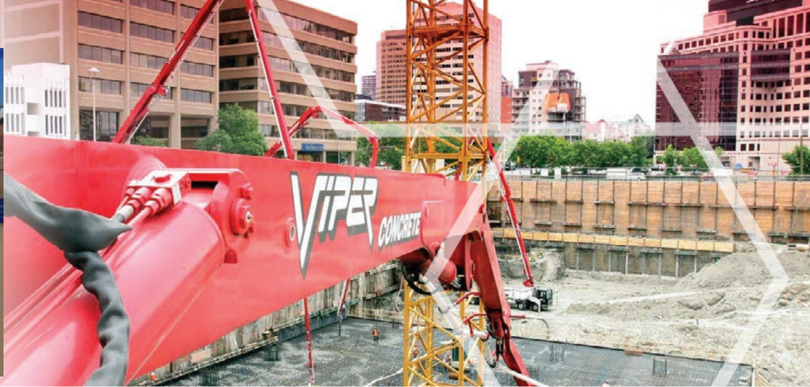
Viper Concrete mass raft pour at Centennial Place. Photo provided by Viper Concrete
